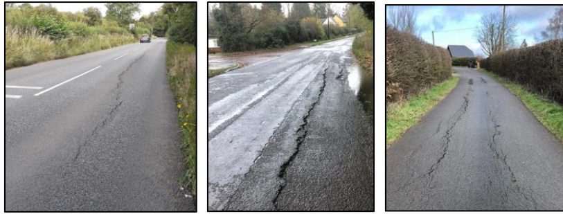
Examples on of longitudinal cracking
